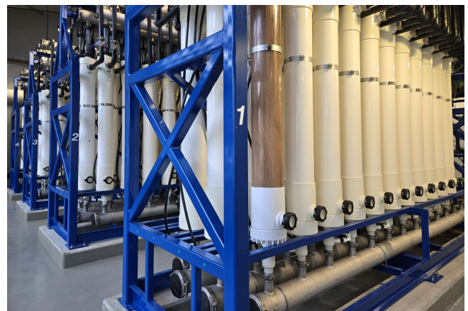
Ultrafiltration Membranes at the water treatment plant
