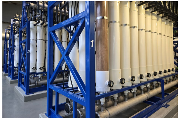
Ultrafiltration Membranes at the water treatment plant
