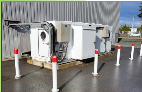
Chemical Room Heating & Ventilation System
