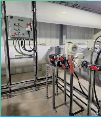
New Flush Water Line Equipment
