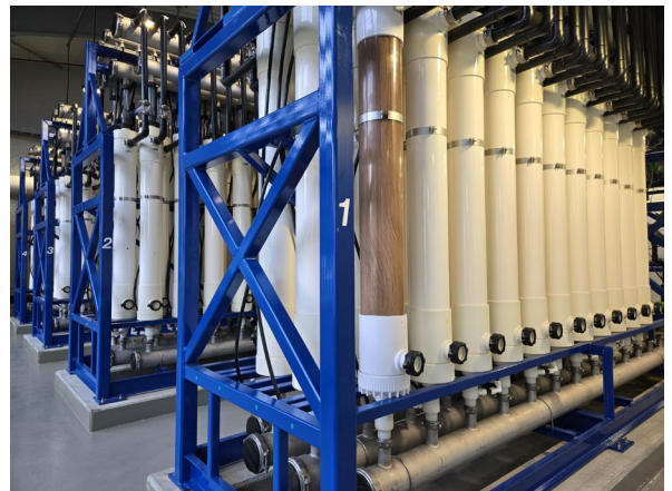
Ultrafiltration Membranes at the water treatment plant
