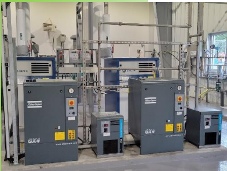
Membrane Air Compressors
