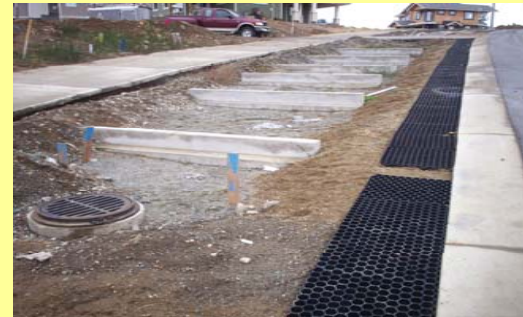
Combination infiltration swale and rain garden project during construction (City of Nanaimo, B.C.).
