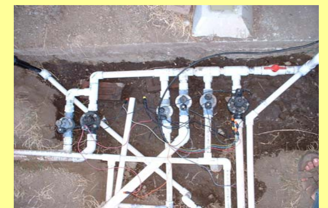
Poor quality design and installation is the most common factor in inefficient irrigation systems
