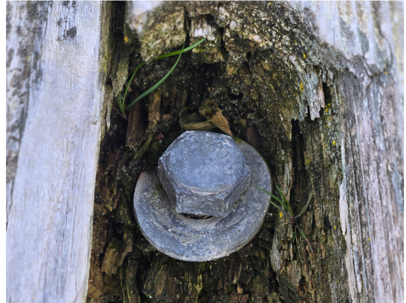
Exposed old lag bolt on bull rail that requires replacement.
