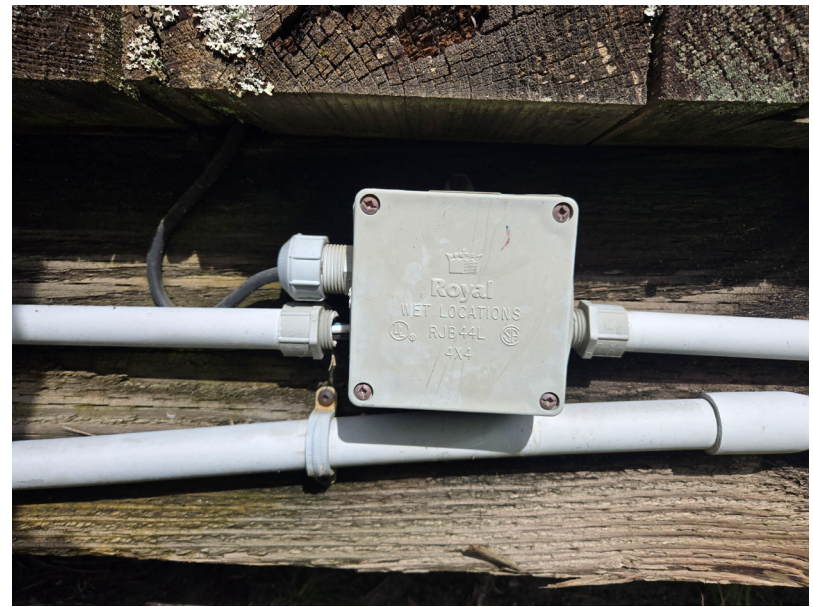
Electrical conduit and junction box behind light fixture on the south face of the boardwalk.
