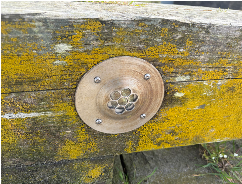
Existing pathway lighting that needs replacement to provide more light. Fixtures are spaced at approximately 30 ft on one side of the boardwalk.
